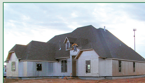
Large custom home with ¾" Reflective-Reflective EPS (RRE) Thermal 3Ht insulation over OSB.
