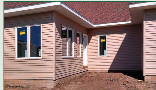
Thermal 3Ht installed under siding of this Cedar Falls, IA home with 3 pictures below.
